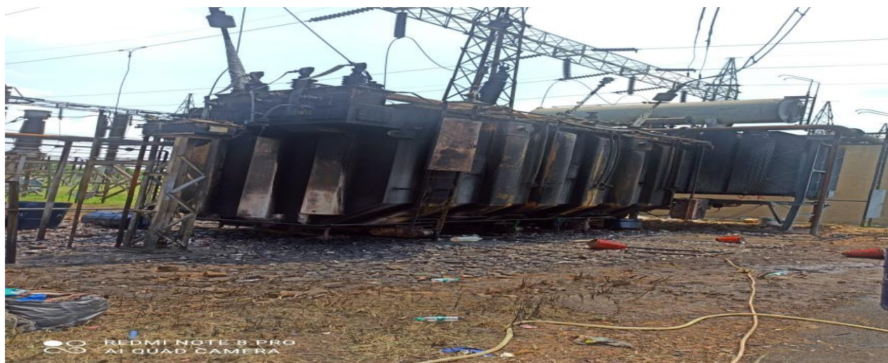
BHEL make Transformer caught fire due to internal fault.
