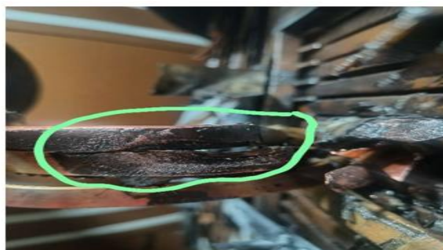
2 No's of winding conductors were melted
