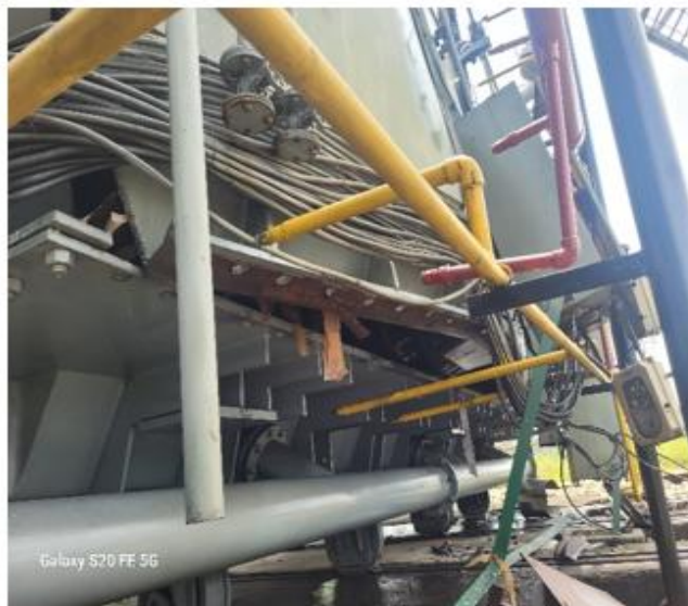
220kV Side main tank
