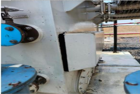
Main tank ruptured & cracks observed at stiffeners
