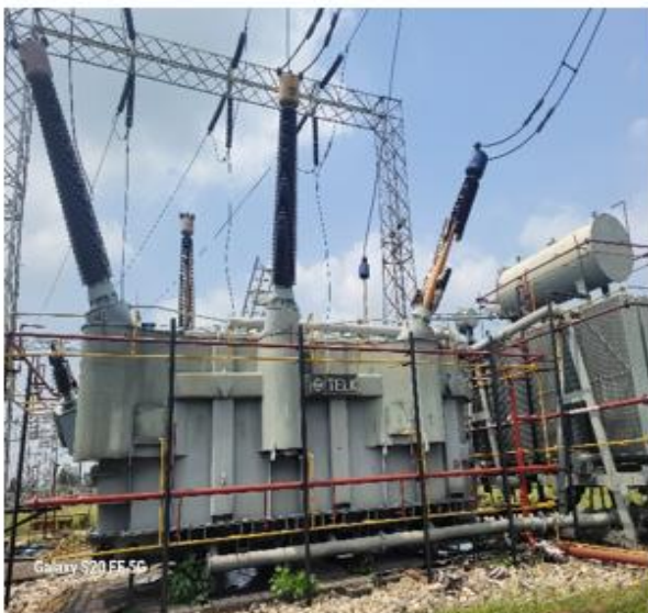
400kV B-Phase Bushing damaged
