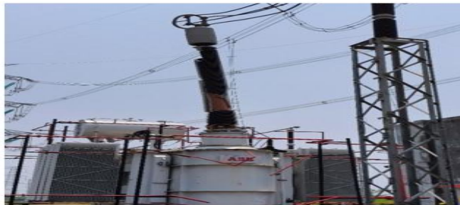
Physical damage of HV bushing
