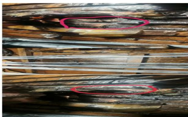
4No's disc layer conductor were found melted
