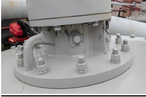
Crack in 220 kV -Phase bushing flange
