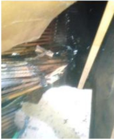
Bulging observed on B-phase HV winding conductors
