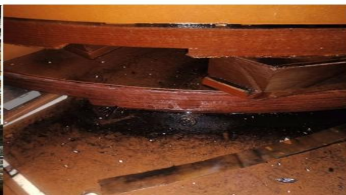
Black marks were observed on below the HV winding lead take off.
