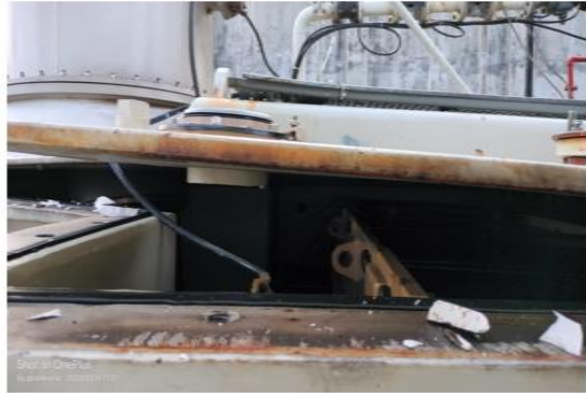
Top side main tank ruptured near HV bushing.
