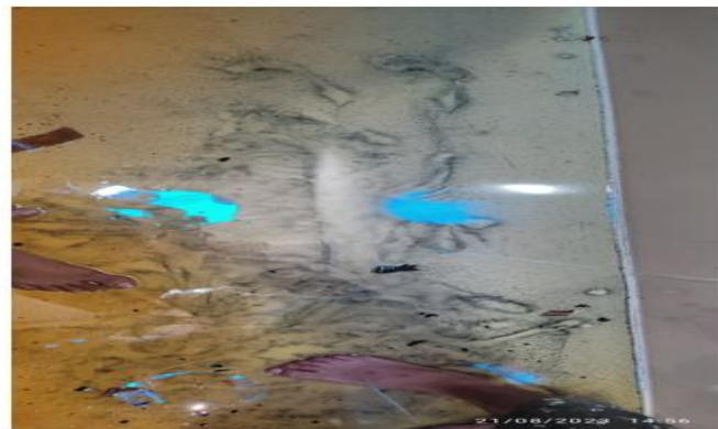
Carbon Powder on tank floor
