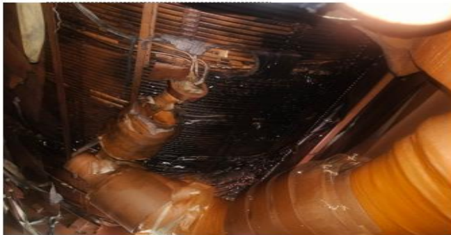
HV lead take out was found dislocated
