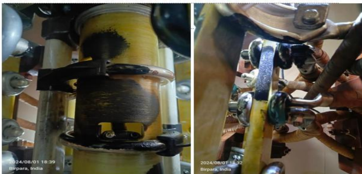
Flash mark on Y-Ph OLTC selector switch
